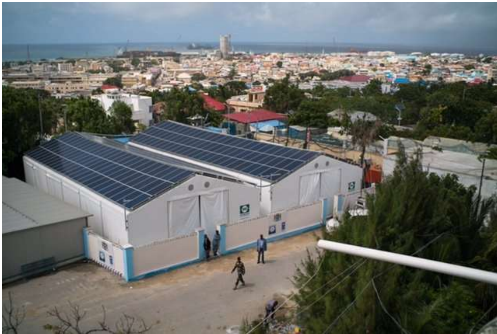
Affordable, reliable and sustainable energy installed at Villa Somalia by UNDP Somalia
